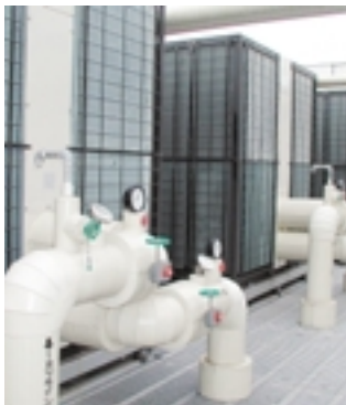
Thermal storage air-conditioning system
