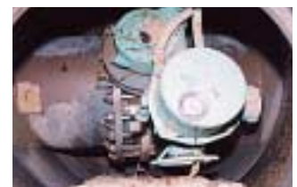
Emergency shutout valve
