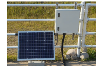
Remote monitoring device panel and solar panels
