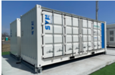
Storage batteries at the Tohoku Site
