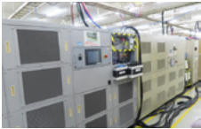
Regenerative power supply test equipment
