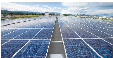
Solar power generation facilities
