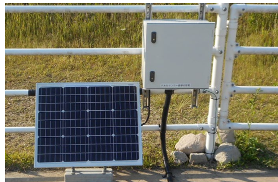
Remote monitoring device panel and solar panels
