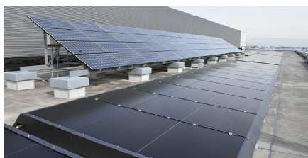
Solar power generation facilities
