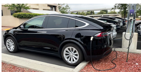
Recharging equipment in a parking area
