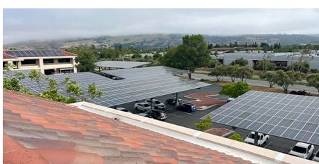
Solar panels on the carport
