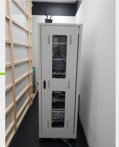
5G base station equipment
