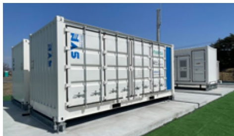
Energy storage facility
