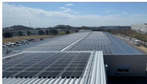
Solar power generation facility
