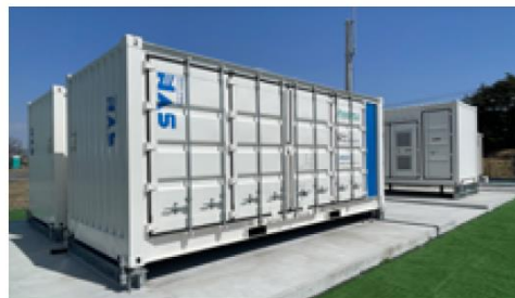
Energy storage facility
