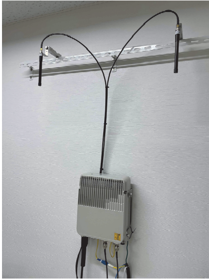
Figure 7 4.8 GHz Band Local 5G Base Station
