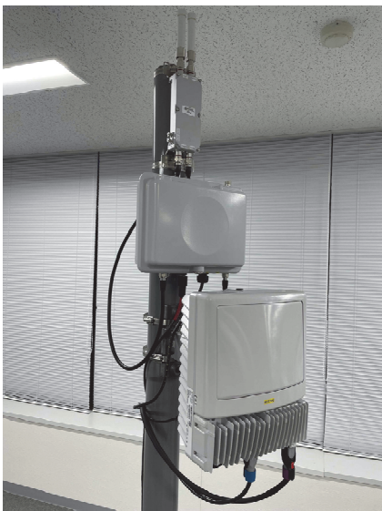
Figure 6 28 GHz Band Local 5G Base Station
