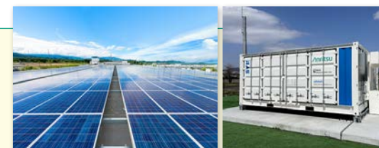
Tohoku Anritsu solar panels (left) and storage batteries (right)
