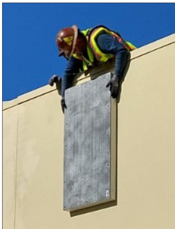
Above figure shows an installation crew placing a cosmetic panel in front of the radio that has been tested to ensure low attenuation in all weather conditions.
