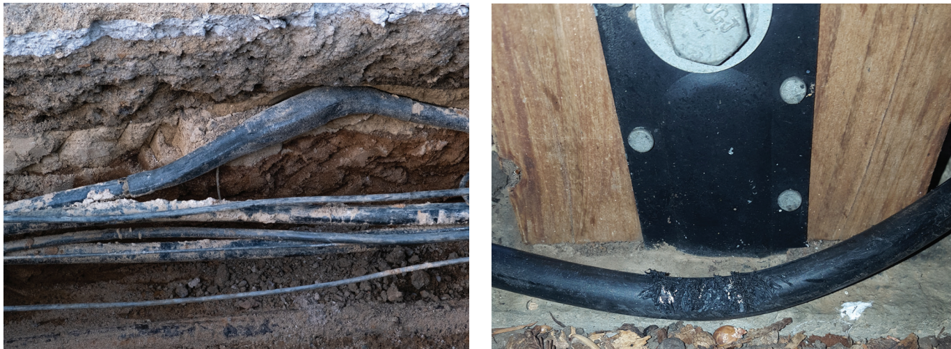
Figure 4. The Insulation of Buried Cable TV Cables and Their Amplifiers can Degrade with Time, or be Gnawed by Rodents as Seen in the Right Hand Image. Breakdown of the Insulation Results in Radiating Interference in Residential Neighborhoods
