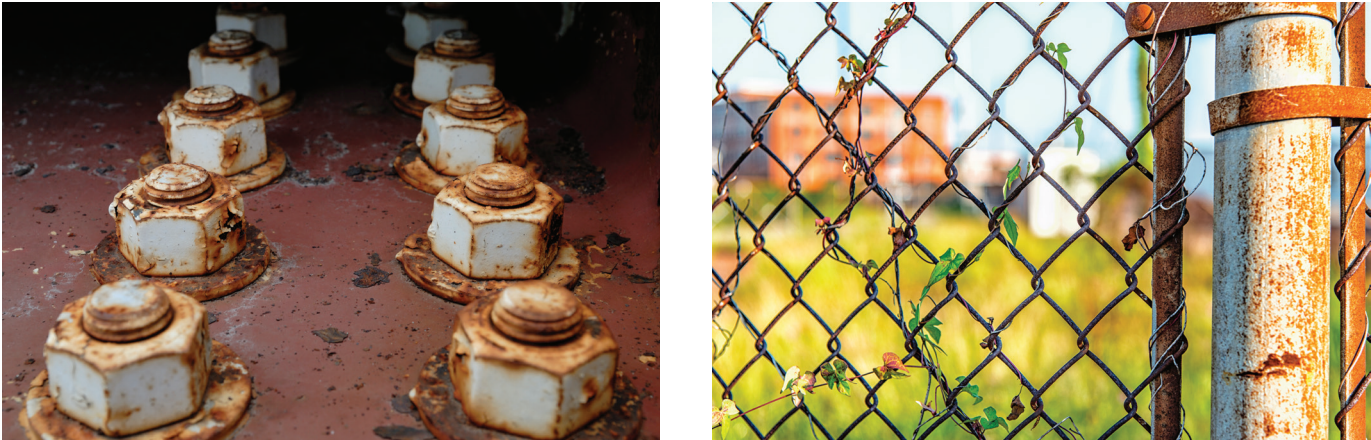
Figure 8. Rusty Bolts and Corroded Metallic Surfaces Generate PIM and Intermodulation Products When Located in Front of Transmitter Antennas
