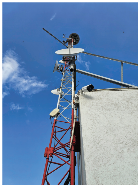
Figure 3. At the Top of this Tower Located on the Highest Building in Kingston Jamaica is an AOA and TDOA Receiver. There are 12 Similar Sites Around Jamaica, All Interconnected to the Headquarters in Kingston.
