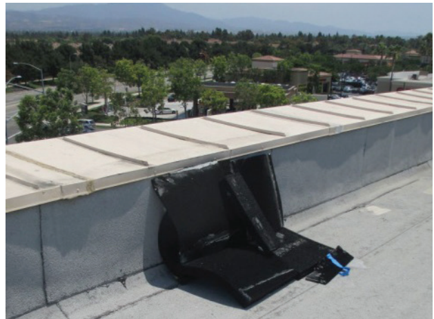
RF Absorber Placed over Small Area Generating PIM
